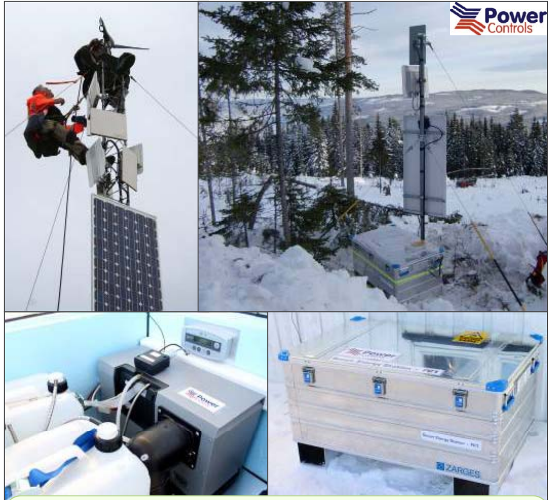
Internet via Radio Link Mast, EFOY Pro in Insulated Outdoor Box (Norway)
