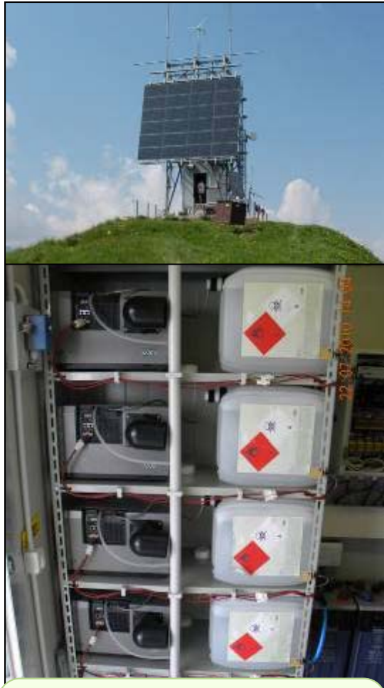
Base Transceiver Station TETRA Radio (Italy)
