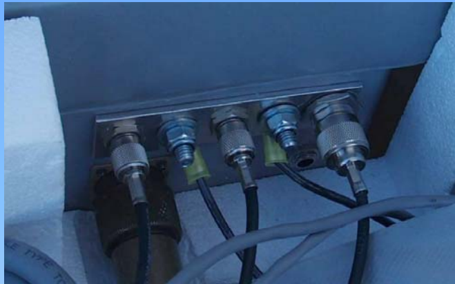
Ground plate and leads inside enclosure
