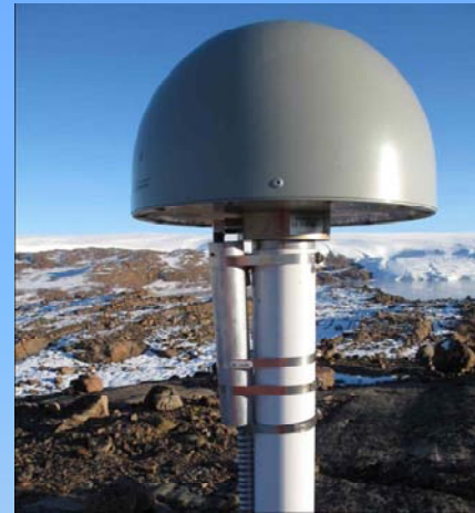
GPS antenna with armored cable and exit point
