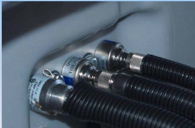
Surge suppressors outside enclosure
