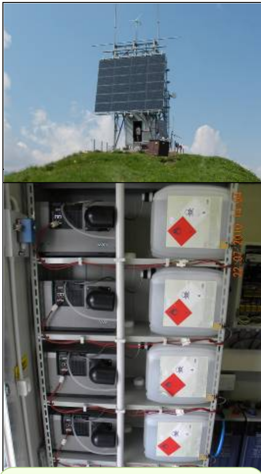
Base Transceiver Station TETRA Radio (Italy)
