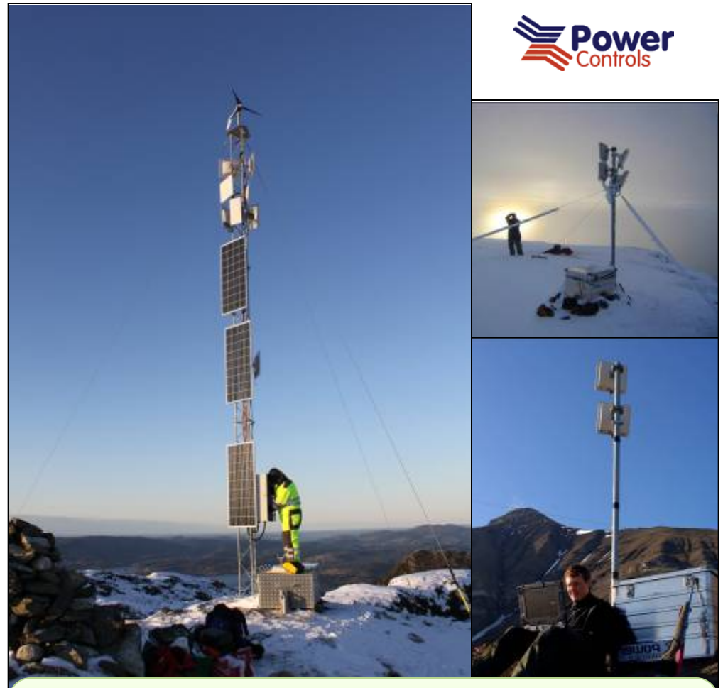
Repeater Stations EFOY Pro in Insulated Outdoor Box (Norway)
