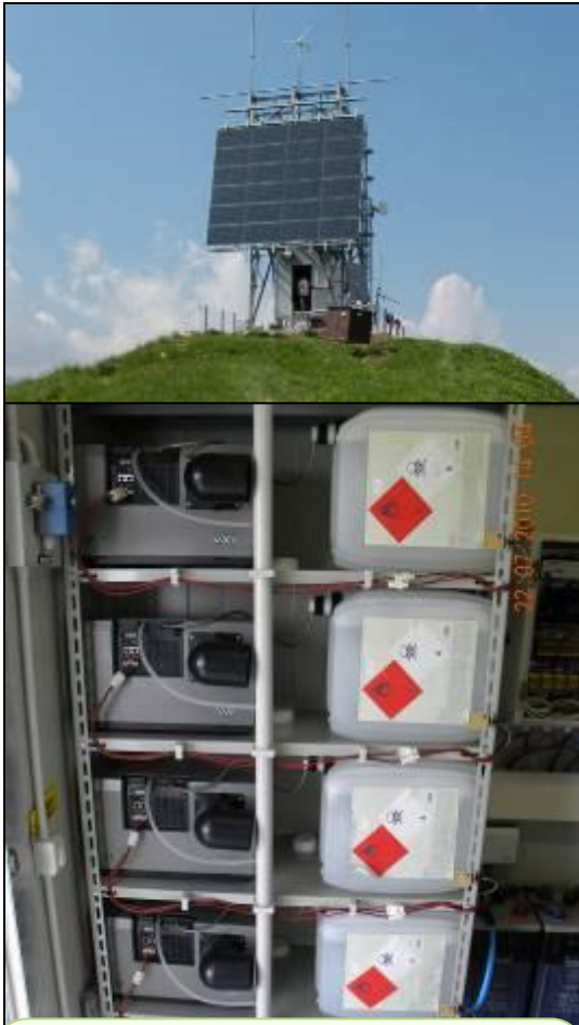
Base Transceiver Station TETRA Radio (Italy)
