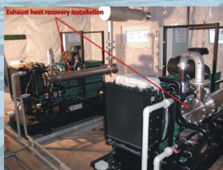
Exhaust heat recovery installation
