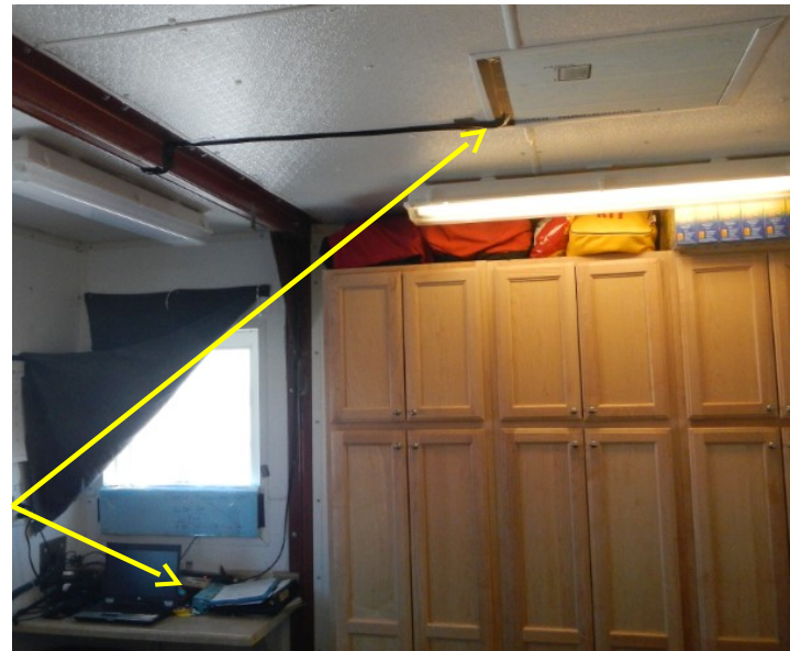
Temporary installation System on table behind laptop Antenna mounted in skylight
