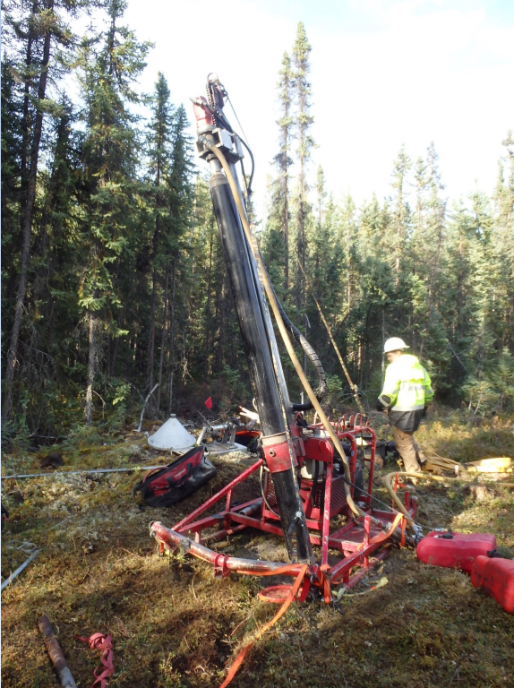
Broken drill rig at I26K
